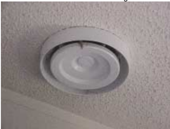
Ventilation fan (utility room and msbath)
