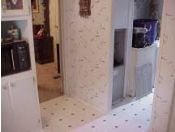
View of AHU and ms floor register
