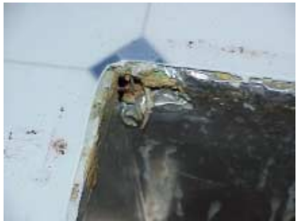
Small duct leak at duct riser (kitchen)
