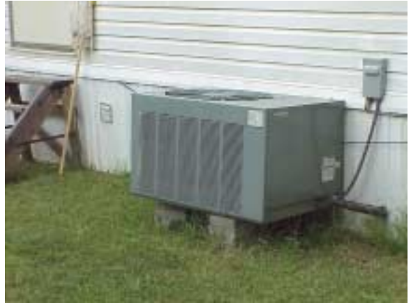
Air conditioner condensor unit
