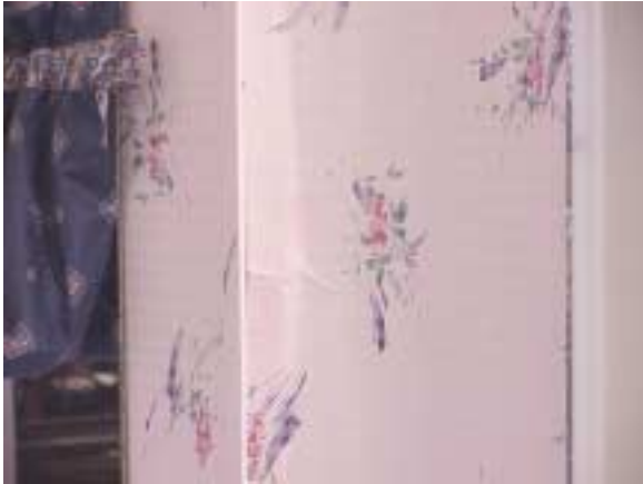
Master bath wall damage
