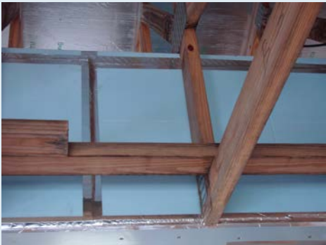
Completed chase, ready for insulation wrap and drywall. Note sealed bottom using 1/2 inch blueboard.
