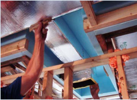
Lateral duct with chase running between trusses. Duct size is limited.
