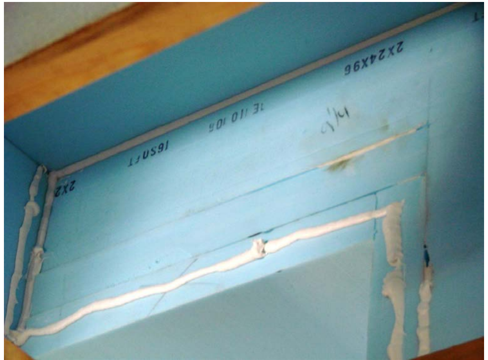
Ready to install the second layer of blueboard. Note the staggered joints and adhesive used to seal seams and attach layers together.
