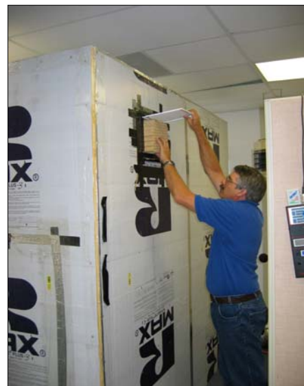
Figure 82 Installing sound baffled return air flow through wall insert made by Tamarack.
