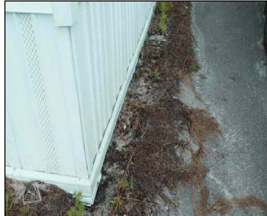
Figure 41 The downstream exit for the water draining across the site via the crawl space. Note flow pattern away from house.
