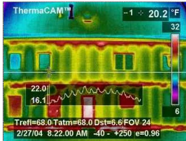
Figure 12 IR-scan showing metal trusses in precast walls. Temperature at the crosshairs is 20.2°F. Overlaid temperature graph shows temperature variation of the surfaces at the white line running horizontally through the crosshairs.
