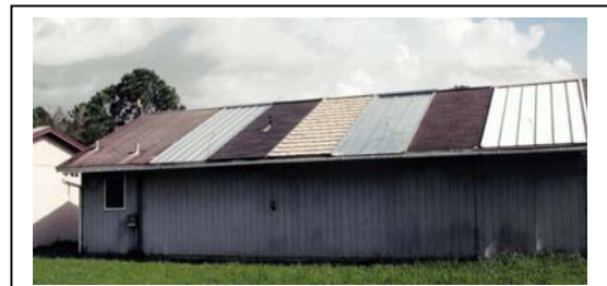
Figure 75 Flexible Roof Facility in summer 2002 configuration. Cells are numbered from left to right starting with the second cell in from the left.
