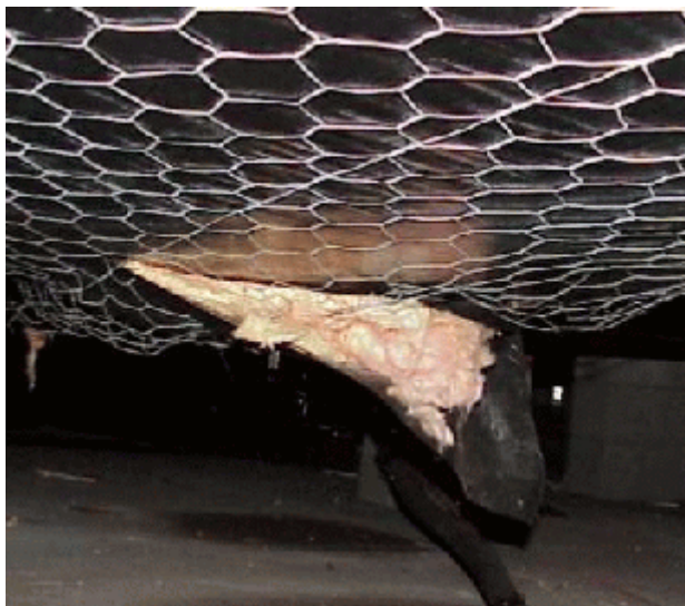
Figure 24. Another belly tear found during inspection.
