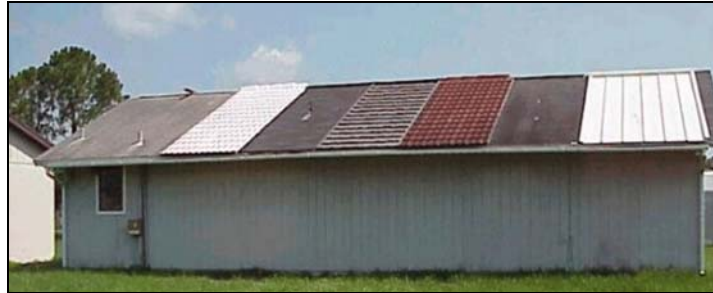
Figure 77 2001 Experimental roof cell. Cells are numbered from left to right starting with the cell second in from the left.
