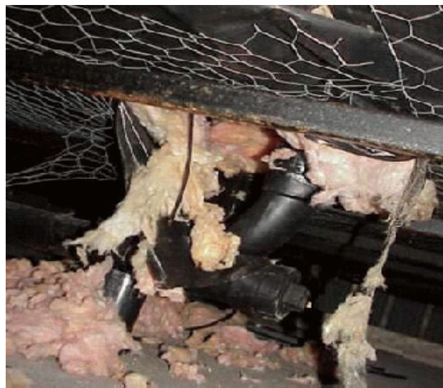
Figure 25 Worst belly tear near plumbing penetration.
