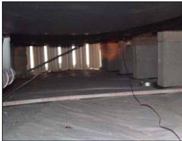
Figure 42 HUD Code required perforations in skirting may not allow adequate volumes of ventilation, creating higher than usual vapor pressure difference across the floor assembly even though the ground cover and belly board are in good condition.
