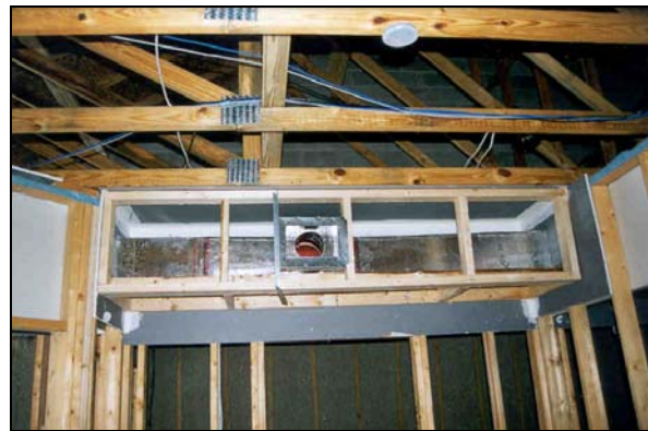
Figure 21 Interior duct system under construction at Lewis Place – the first Energy Star apartment complex in the country.
