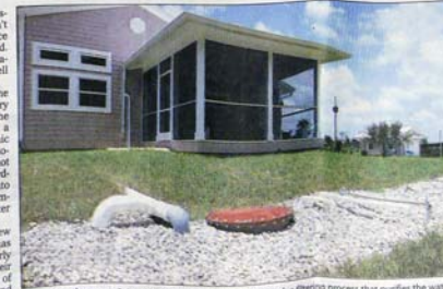
Water from heavens. Rainwater flows to a cistern, then through a filtering process that purifies the water.
