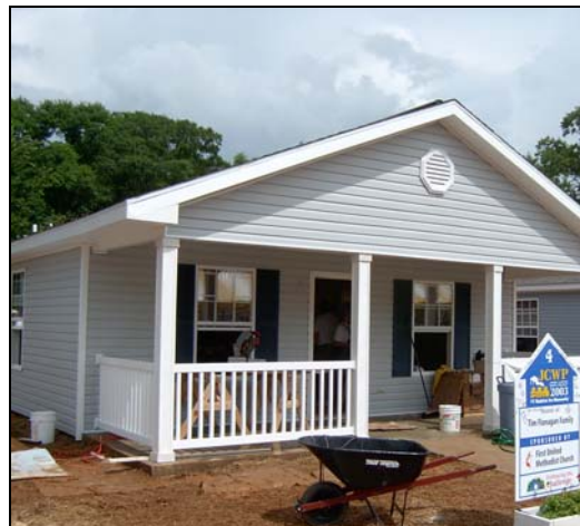
Figure 17 2003 Jimmy Carter Work Project house in LaGrange GA – one of 22 Energy Star homes built in one week.
