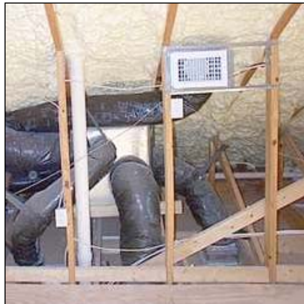
Figure 60 semi-conditioned space for the ductwork.
