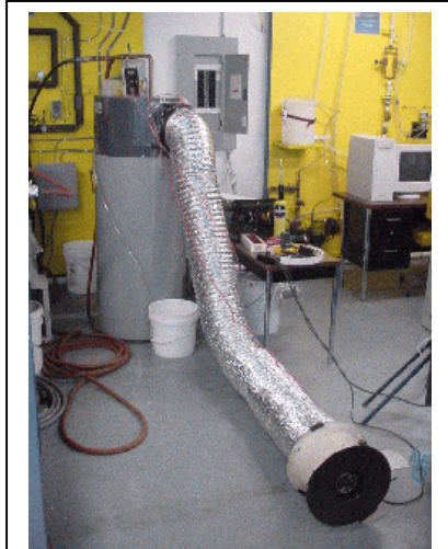
Figure 87 Airflow measurements using a Duct tester on heat pump cold air discharge side.
