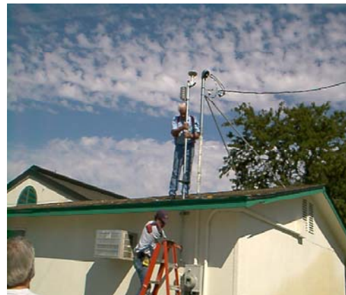
Figure 55 Weather monitoring system installation in the Boise portable classroom.
