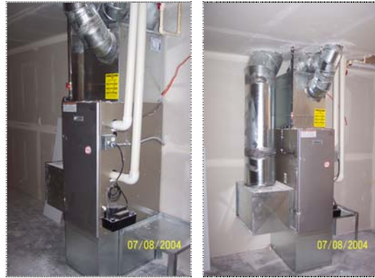
Figure 33 90% AFUE Furnace, as installed at Kokanee Creek
