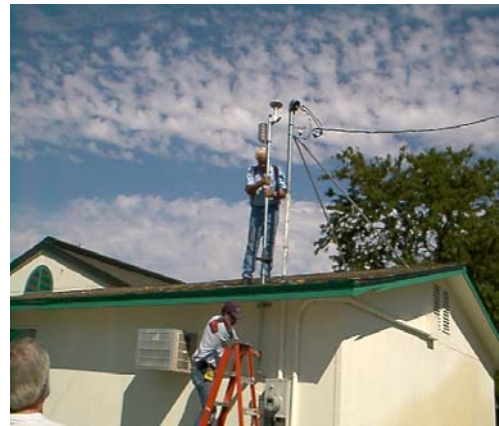
Figure 67 Weather monitoring system installation in the Boise portable classroom.
