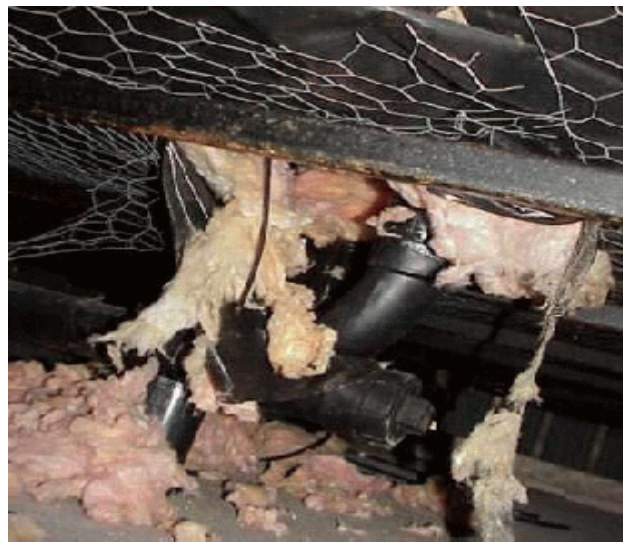
Figure 37 Worst belly tear near plumbing penetration.
