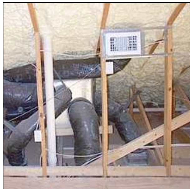
Figure 73 semi-conditioned space for the ductwork.
