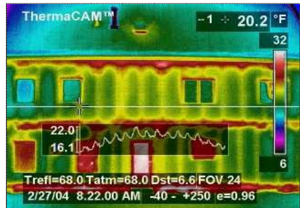
Figure 14 IR-scan showing metal trusses in precast walls. Temperature at the crosshairs is 20.2°F. Overlaid temperature graph shows temperature variation of the surfaces at the white line running horizontally through the crosshairs.
