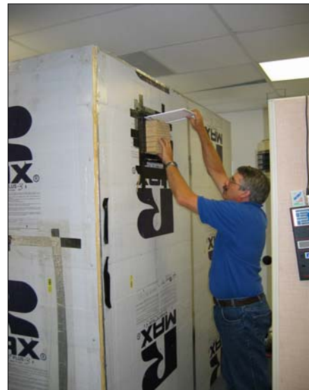
Figure 96 Installing sound baffled return air flow through wall insert made by Tamarack.
