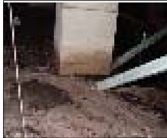
Figure 50 Flow lines under house, indicating running water under the house. Also note the “tide line” on the support column.
