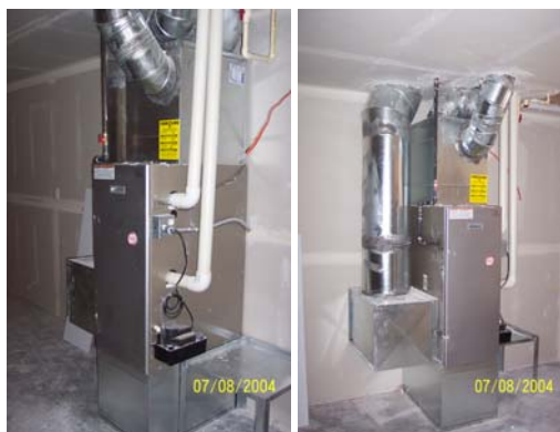
Figure 5 90% AFUE Furnace, as installed at Kokanee Creek
