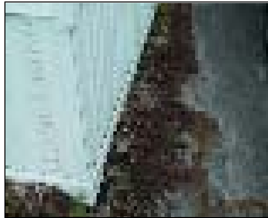
Figure 51 The downstream exit for the water draining across the site via the crawl space. Note flow pattern away from house.
