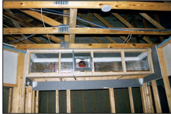
Figure 27 Interior duct system under construction at Lewis Place – the first Energy Star apartment complex in the country.
