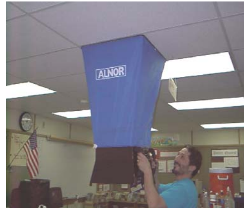
Figure 66 Ventilation system testing at North Thurston School District.
