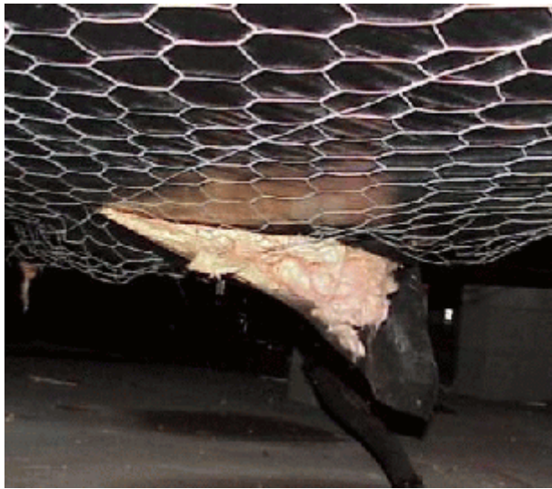
Figure 36 Another belly tear found during inspection.
