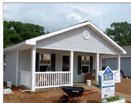
Figure 23 2003 Jimmy Carter Work Project house in LaGrange GA – one of 22 Energy Star homes built in one week.
