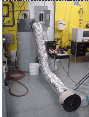
Figure 100 Airflow measurements using a Duct tester on heat pump cold air discharge
