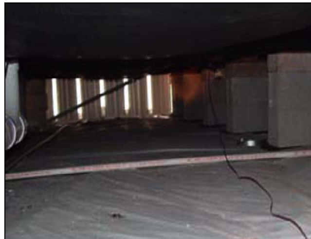
Figure 52 HUD Code required perforations in skirting may not allow adequate volumes of ventilation, creating higher than usual vapor pressure difference across the floor assembly even though the ground cover and belly board are in good condition.
