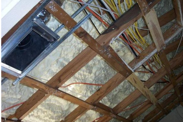
Figure 6 Sealed attic with spray foam insulation (Icynene™). Note the duct work is below the insulation, which places it within the air & thermal boundaries.
