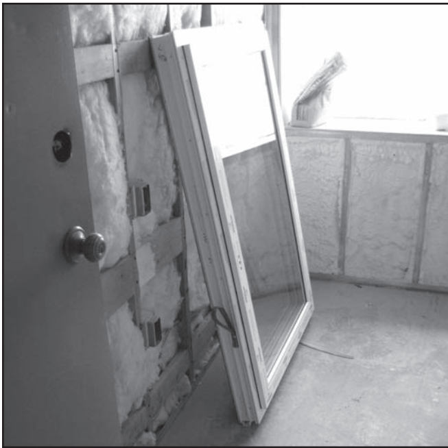
Figure 2. High performance windows prior to installation. The team had to calculate minimum projection of drip edges and overcome rowlock brick sill details to make sure window installation would be durable. The team ran metal flashing beyond its normal point on the upper face to better protect the sill brick by going past the top surface of rowlock. Photo courtesy Michael Whartnaby of Thoughtful Balance, Inc.
