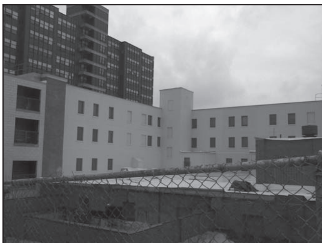
Figure 6. A photo of the rear section of the building. In confronting performance in retrofits, addressing unique details inherent to the building are vital. Photo courtesy Michael Whartnaby of Thoughtful Balance, Inc.
