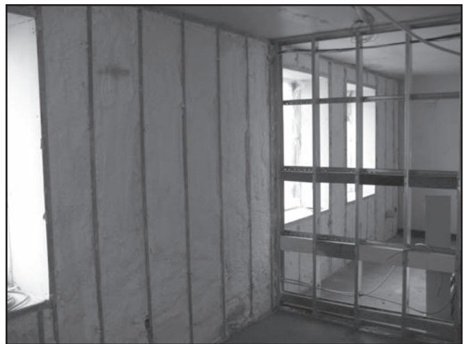
Figure 4. The most common wall at McKeesport YMCA, an existing wall of 14" thick masonry, with the addition inside of an additional 8" close cell spray foam. The typical wall is now an R-57. Photo courtesy Michael Whartnaby of Thoughtful Balance, Inc.
